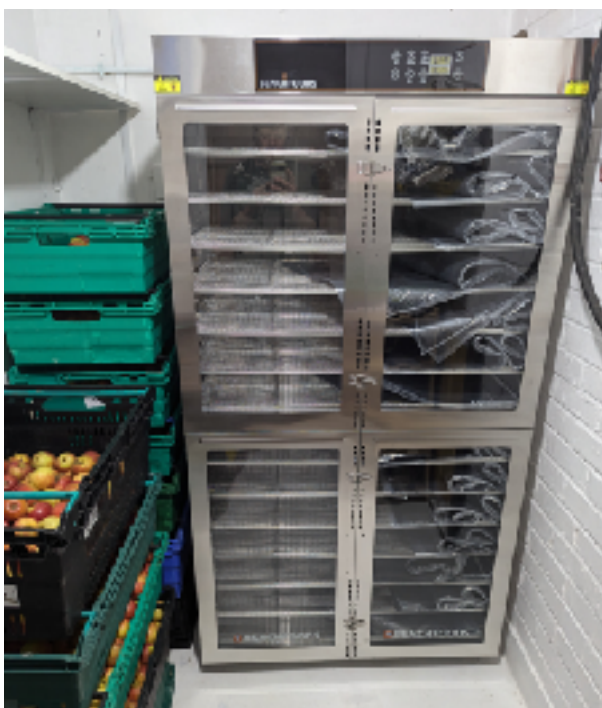
Our first dehydrator installed at The Well
